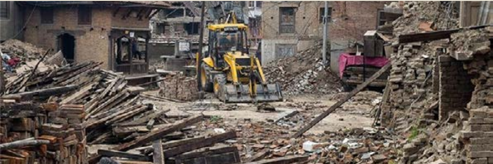
One of the biggest impediments to reconstruction has been the slow pace of clearing debris and demolishing irreparable buildings .
