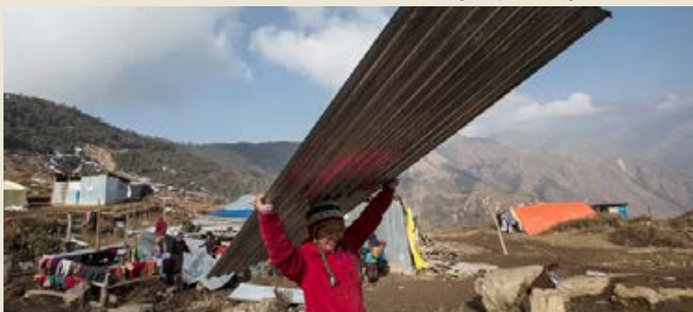
A woman carries a metal roof panel to rebuild her damaged house in Laprak, in Nepal's Gorkha district.
