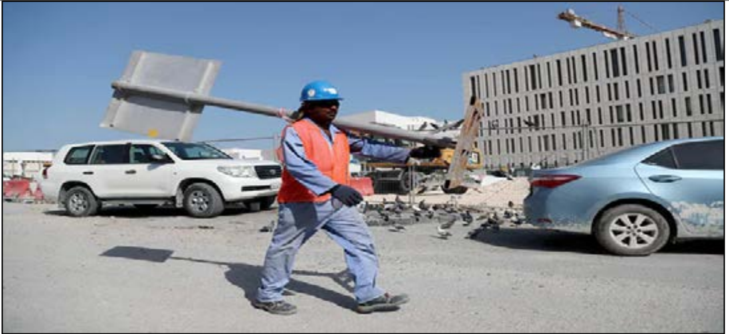
A migrant worker carries a pole at a World Cup construction site in the Qatari capital Doha.
