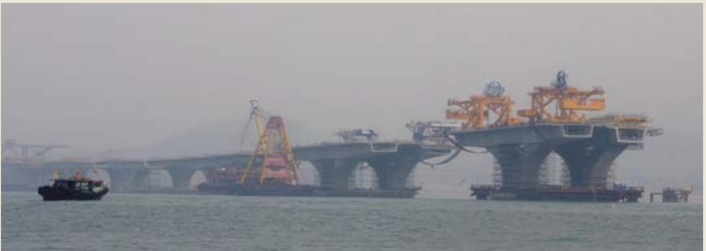
The concrete tests were carried out on the Hong Kong-Zhuhai-Macau bridge project.
